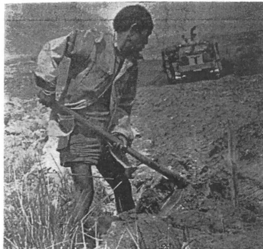
'SELF HELP' — A Montagnard villager lends a hand on a recent brigade civil affairs project near Khanh Duong where the brigade conducted Operation Summerall. The villager is helping build a fish pond that will serve as a protein diet supplementary for the Montagnards.
