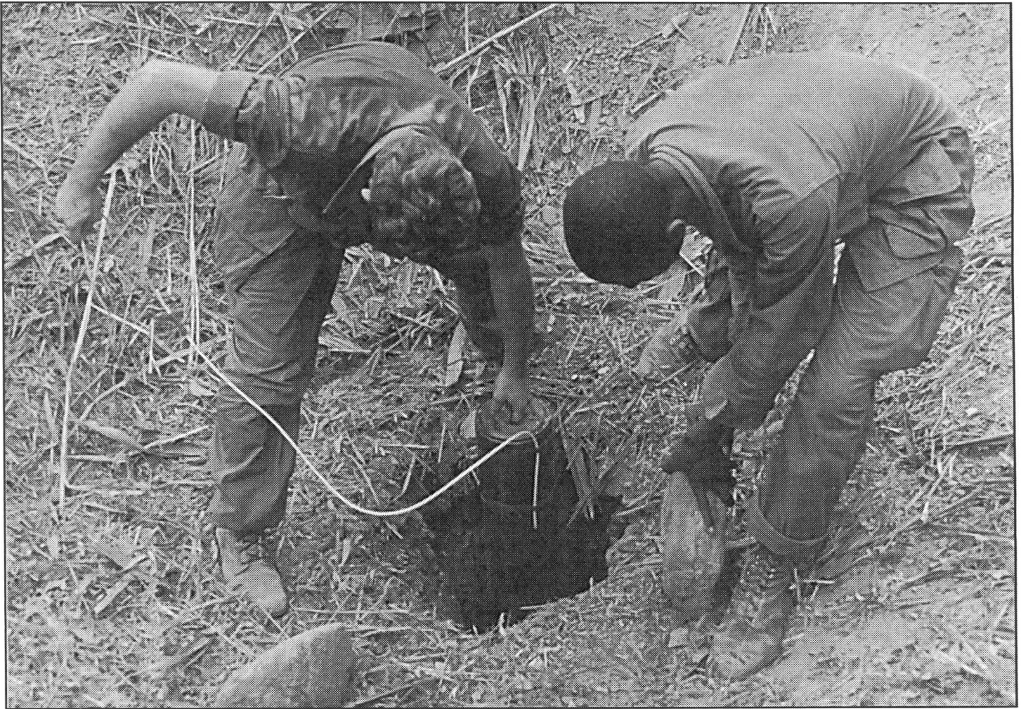
CNU LAI, Vietnam--TUNNEL BUSTERS. Spec.4 Logan E. Harris, Brooksville, Fla., and Pfc. Moses Tasto, Eutawville, S.C., lower an explosive charge into a VC tunnel discovered near here during Operation Benton. Both men are assigned to A Co., 326th Engineers, 101st Airborne. (USA Photo by SSG Art Campbell)
